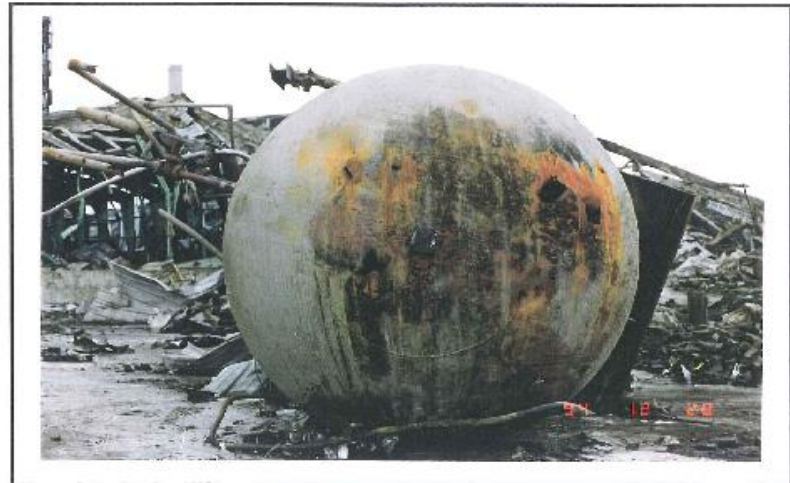
Photo 8 - 13 Ammonia Bullet Tank Damage
